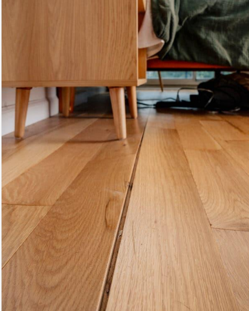
Building defects caused buckling floors.Credit...Clark Hodgkin for The New York Times Image
