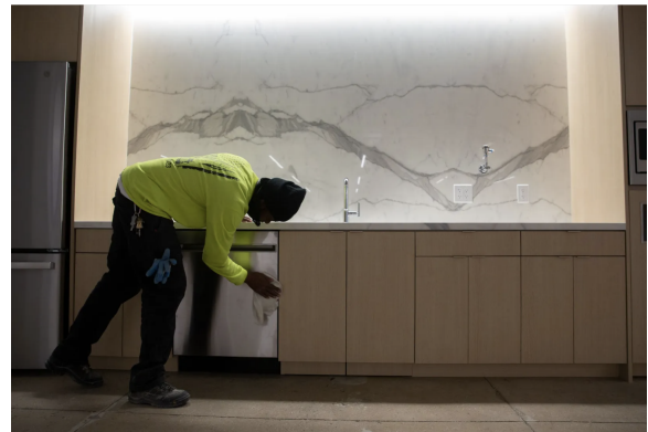
A worker buffed new fixtures in a renovated loft-style office space on West 40th Street last week. | Ben Fractenberg/THE CITY
